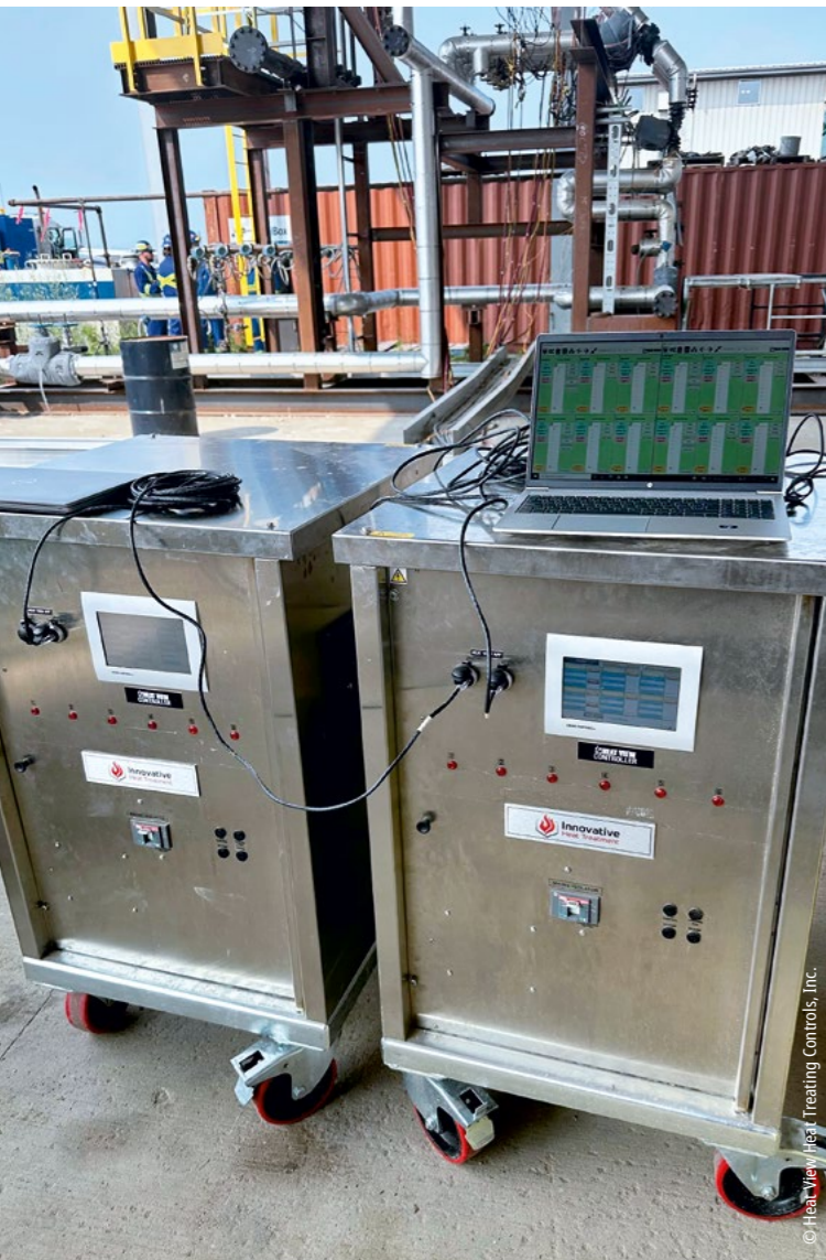
In the embedded version, the Heat View control system is operated via the built-in 7-inch touchscreen of the CP6606 Panel PC.
